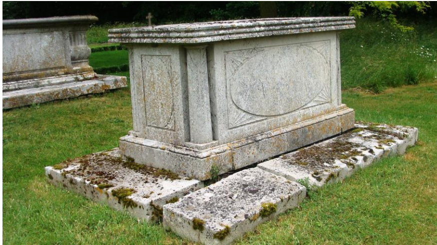
Picture 4. Listed chest tomb within St Mary's churchyard, one of two in need of repair and restoration and both, without prejudice, potentially eligible for EHDC financial assistance.
