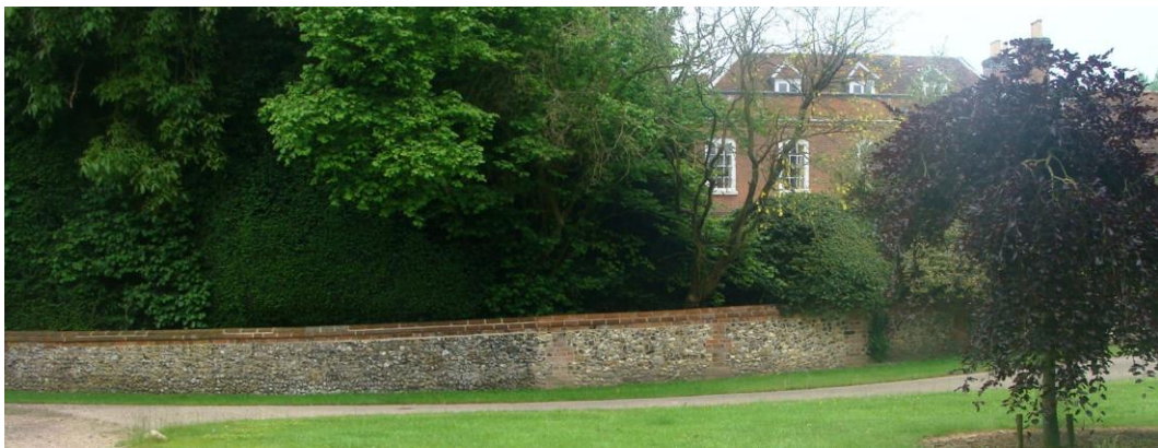
Picture 25. Brick and flint wall recently repaired, important to the setting of Westmill Bury.
