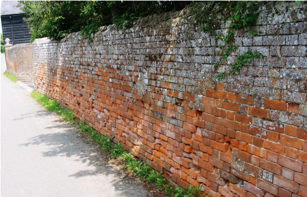
Picture 24. Frontage wall to Dial House. A prominent feature in a key location and in need of repair.
