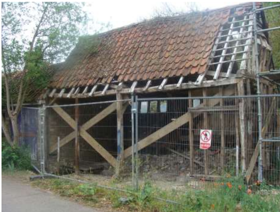
Picture 13- Outbuilding within the curtilage of a Listed Building off White House Close in urgent need of restoration.
