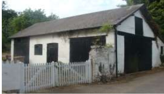
Picture 24 - Outbuilding to Watton Cottage. Selected original wooden doors and associated ironmongery are features worthy of additional protection.
