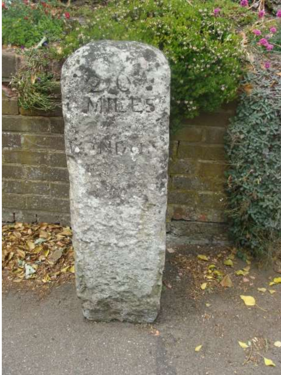
Picture 12 - Listed Milestone, cleaning, general restoration and repainting is recommended. It is included in the Council's Buildings at Risk Register.
