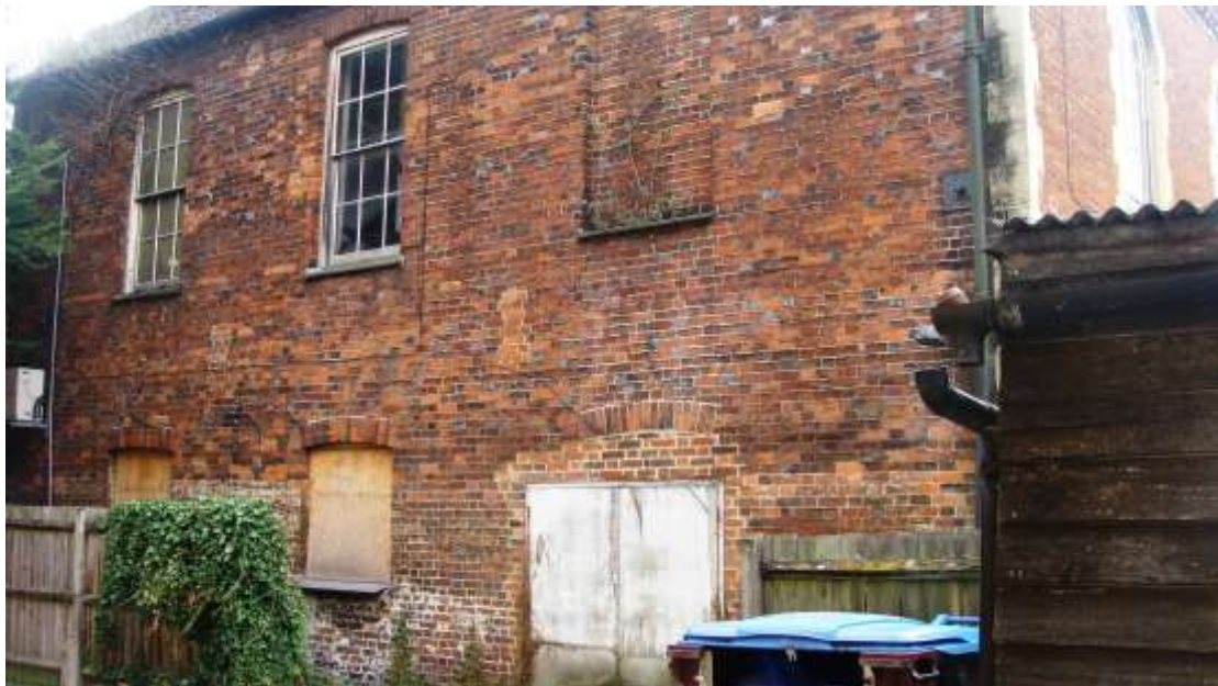
Pictures 12-13. The high quality and deteriorating condition of no. 19 Church Street- building now included on the Council's Heritage at Risk Register.
