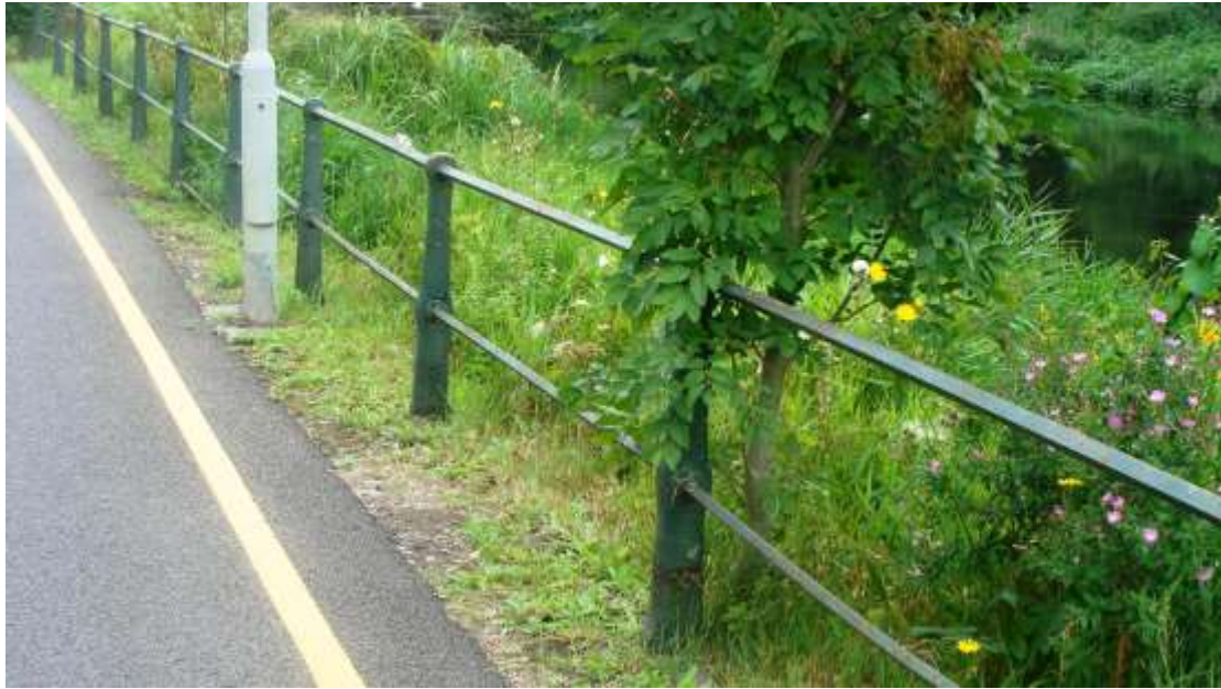
Pictures 112-113. Quality railings of historic importance contribute to the street scene; some sections are in need of repair.
