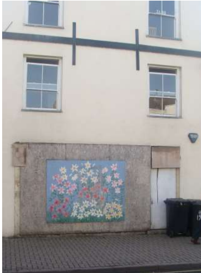
Picture 49. No.19 Amwell End, a building in need of repair and occupation.
