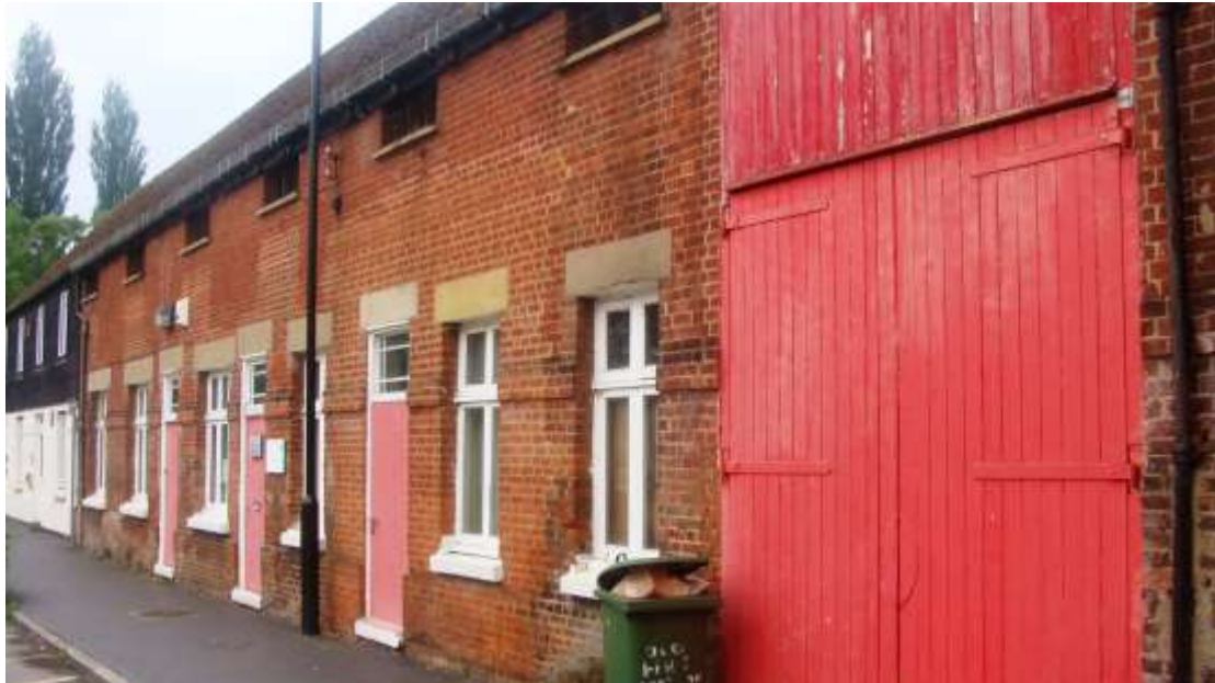
Picture 20. Simple building identified on modern mapping as being 'The Old Fire Station' that should be retained. Some coordinated repainting/refurbishment would be beneficial.
