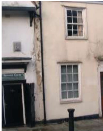
Picture16. Nos.96 - 96A High Street facing onto Tudor Square. Remedial works required.
