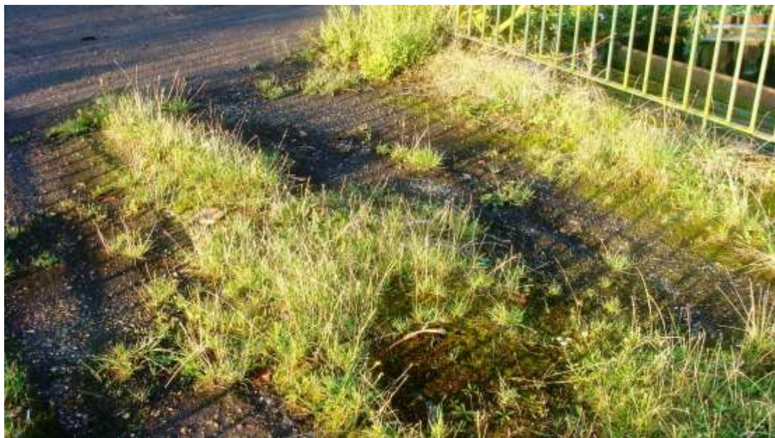
Picture 42. Vegetation on surface to listed bridge Hertford Road in need of removal. It is hoped it remains structurally sound?
