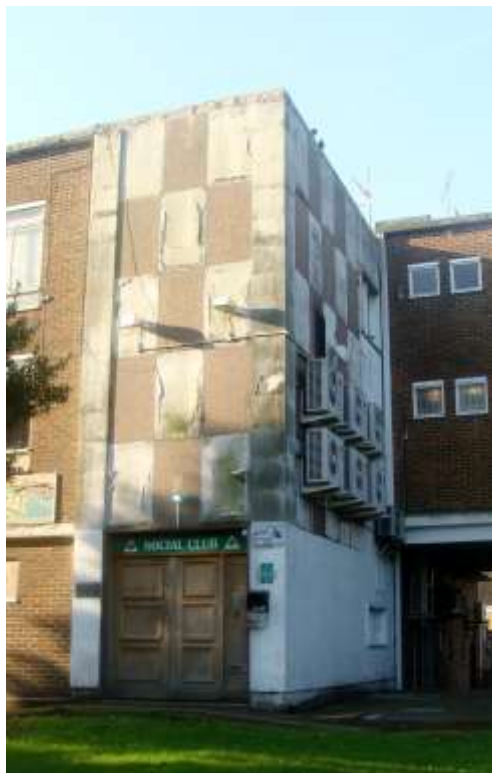
Picture 56. Poor quality building at strategic north western corner of Amwell End whose appearance seriously detracts from the Conservation Area.
