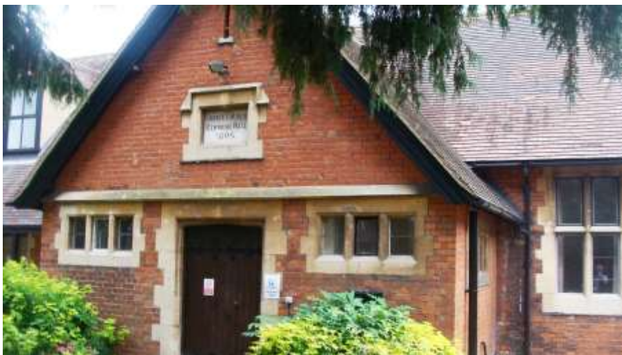
Picture 68. Good quality window and other detailing to Christ Church Memorial Hall, rear of Christ Church, New Road.
