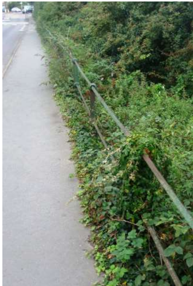
Picture 51. Low railings less than 1m in height and thus unprotected from demolition within the Conservation Area. Potential candidates for formal protection by Article 4 Direction. Need to remove vegetation repair and repaint. In first instance need to discuss issue with Thames Water if indeed they are the owners.
