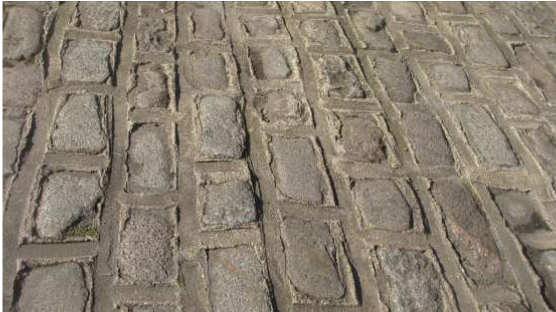
Picture 46. Surface detail adjacent to former Goods Station - a small but important detail.
