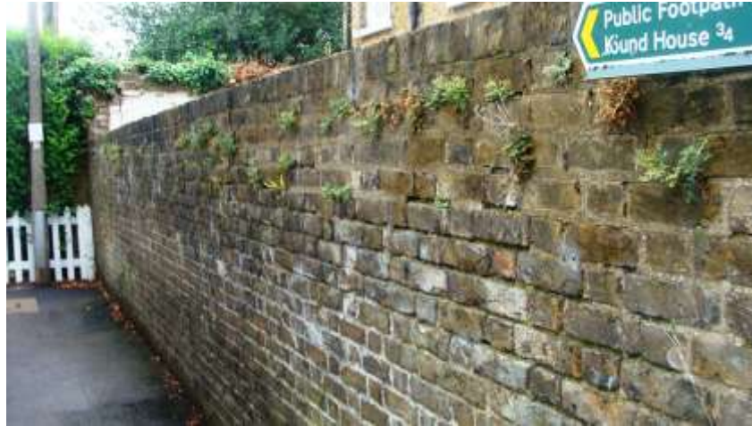
Picture 93. A short but important length of wall adjacent to footpath 5 Little Horse Lane, most worthy of retention.
