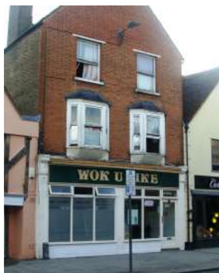
Picture 23. A prominent shop in the High Street in urgent need of restoration and improvement. The dominant nature of the facia detracts.
