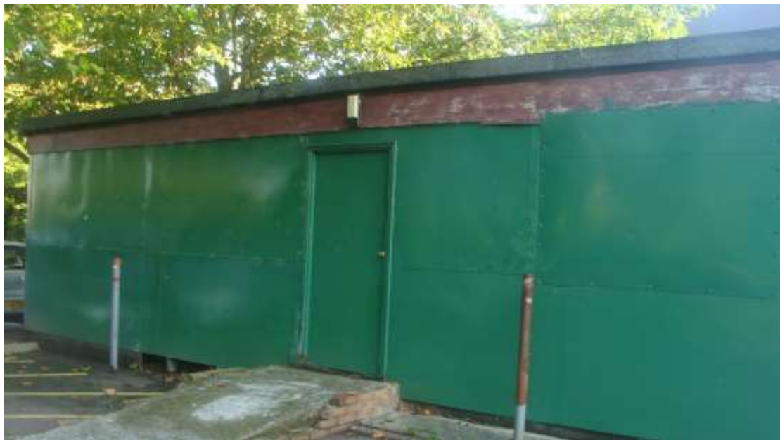
Picture 54. Temporary structure on EHDC car park Broadmeads which detracts. Should be removed or replaced. As a short term measure it needs repainting.
