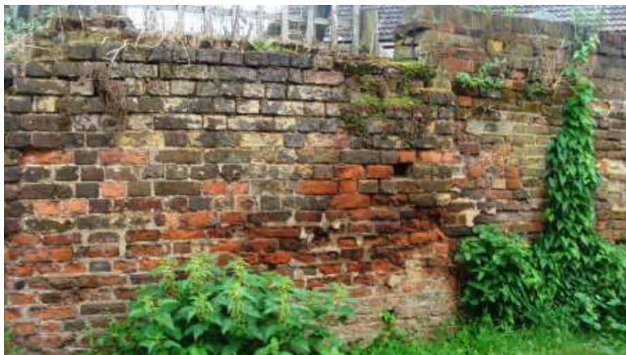
Picture 92. Wall in deteriorating condition to be retained; to rear of South Maltings, New Road.
