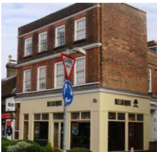
Picture 10. No. 12 High Street. Removed from Register following improvements and occupation of ground floor - condition of upper windows need repairs.
