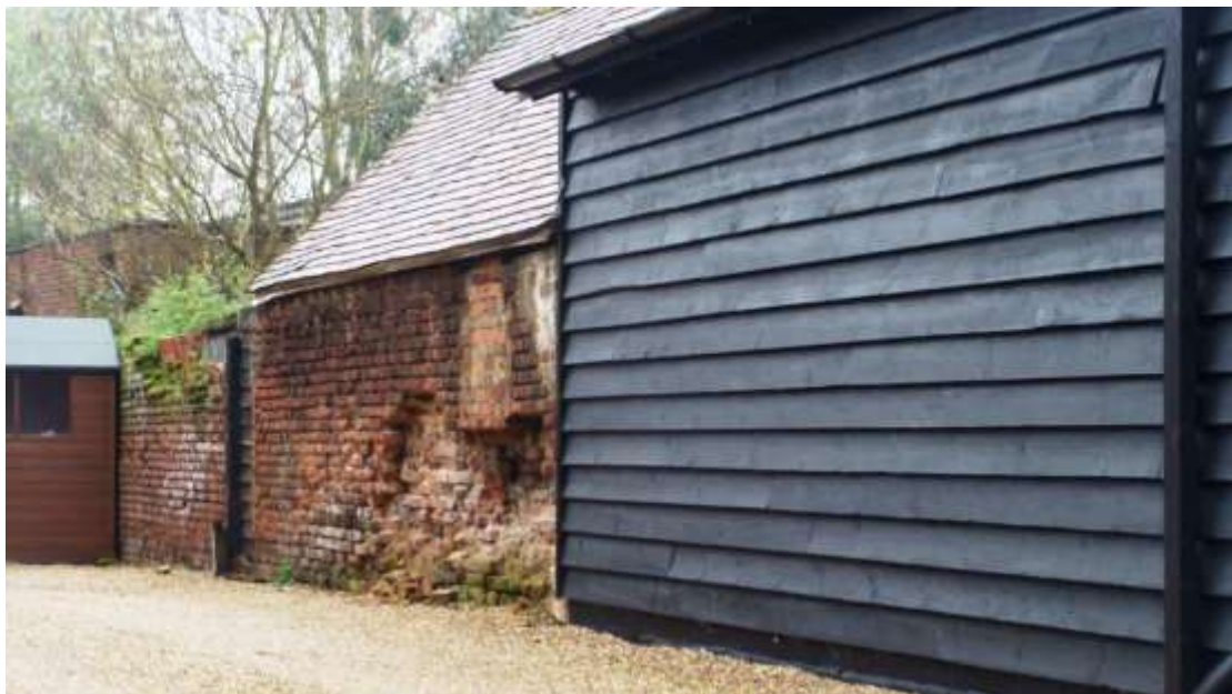
Picture 15. Ancillary building assumed to form part of Trinity Barn complex whose brickwork is in need of repair.
