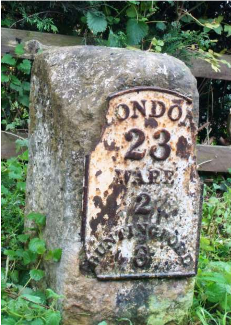
Picture 1. 18th century milestone for Wadesmill Turnpike Trust in need of repair. Included on the Council's Heritage at Risk Register.
