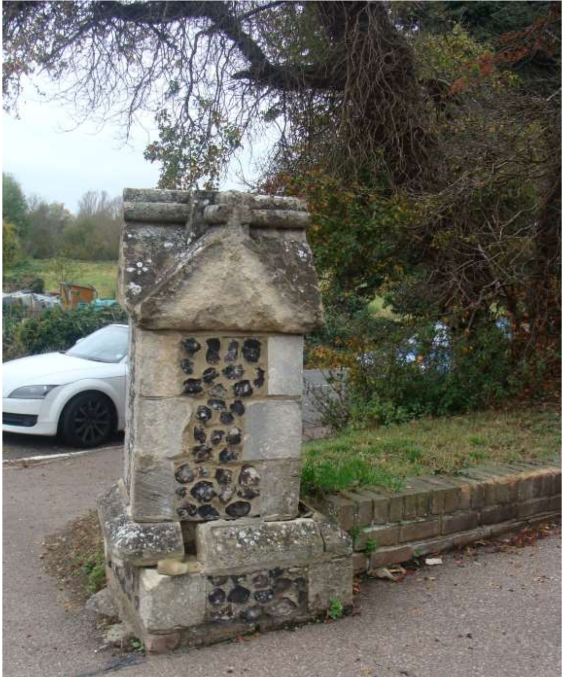
Picture 12 – Individually listed 19 th century grade II pier to St Andrews Church, Cappell Lane, in need of repair. (Subsequently repaired)
