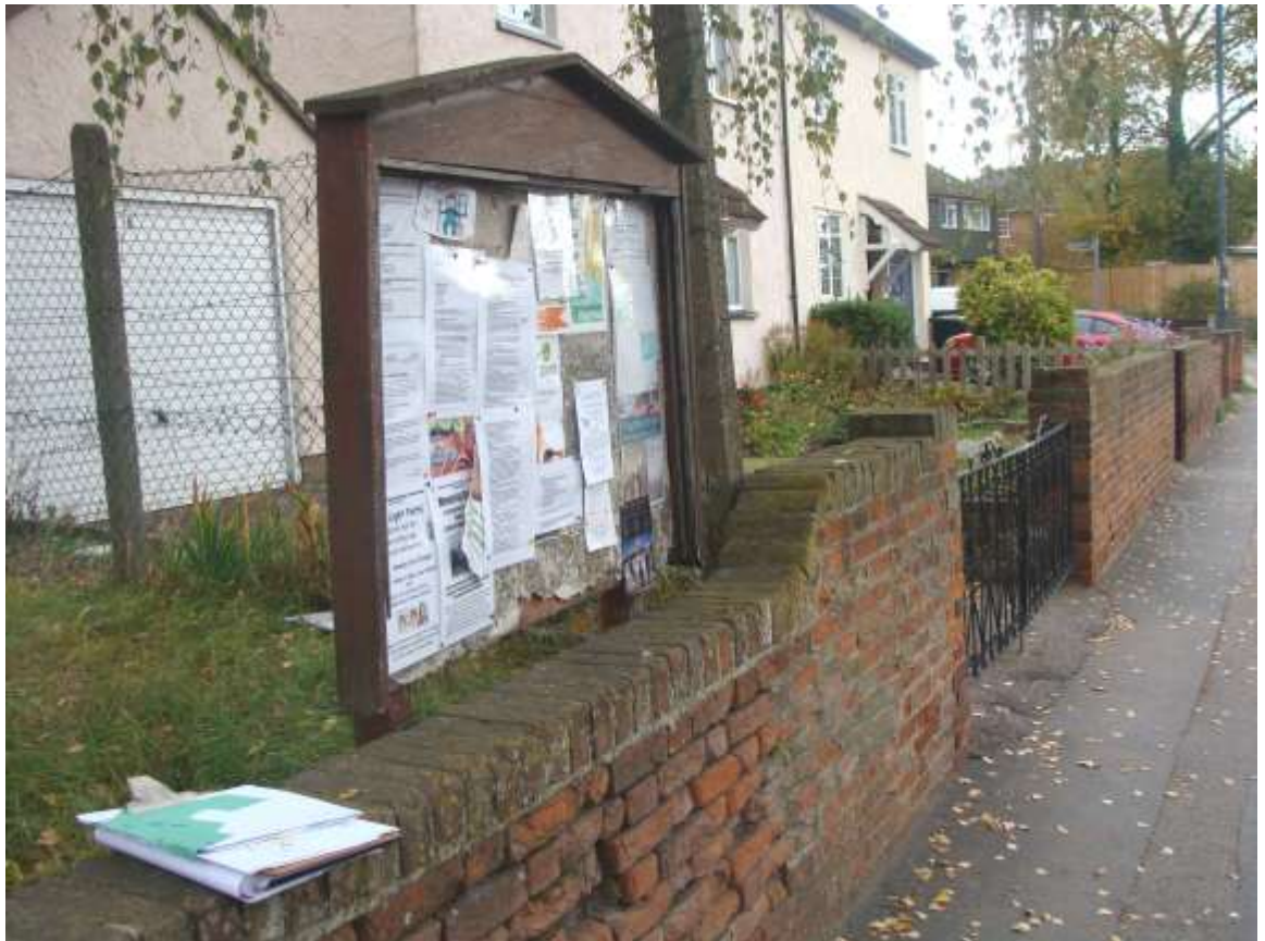
Picture 24 – The area around the Parish Notice board, including wall to front and boundary dividing fence would benefit from general repairs and improvements.
