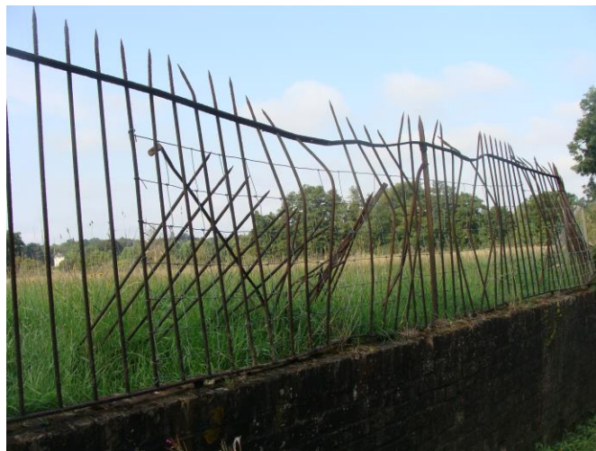
Picture 33- Dilapidated sections of agricultural estate railings to east of Maltings Lane; in need of repair.
