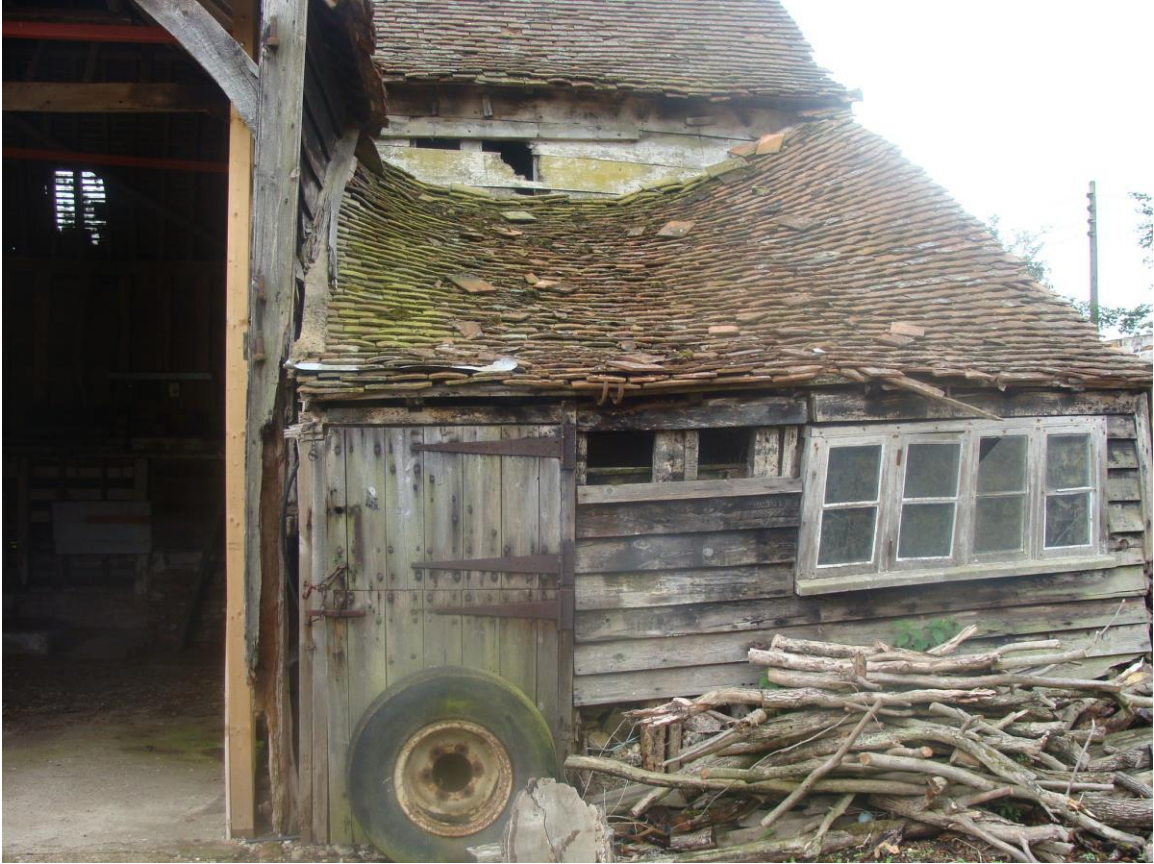
Picture 41- detail of deteriorating condition, comment as caption for Picture 40.
