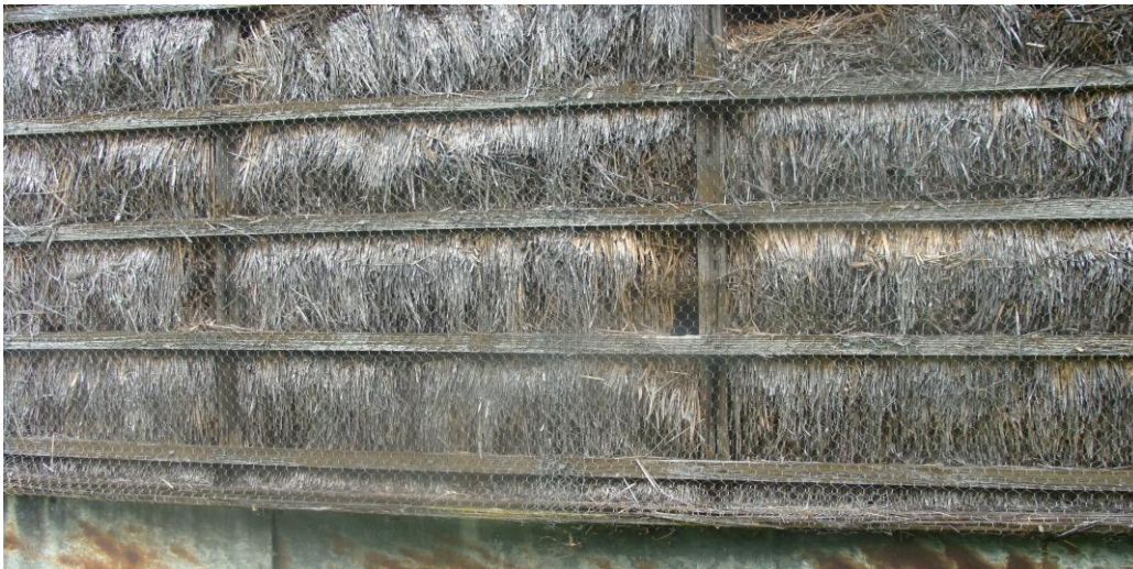
Picture 43- External construction detail of building previously used as a Great War ammunition shed. Most unusual; unclear at present as to whether or not the straw, presumed to be insulation, is contemporary with original use or added afterwards in conjunction with later use as an apple store.
