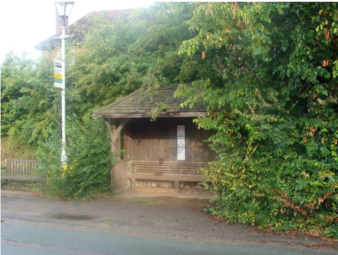
Picture 27- Constructed in 1977 to commemorate Queen Elizabeth's Silver Jubilee, this simple timber framed shelter is well proportioned and constructed. Recent repair works have improved its appearance.
