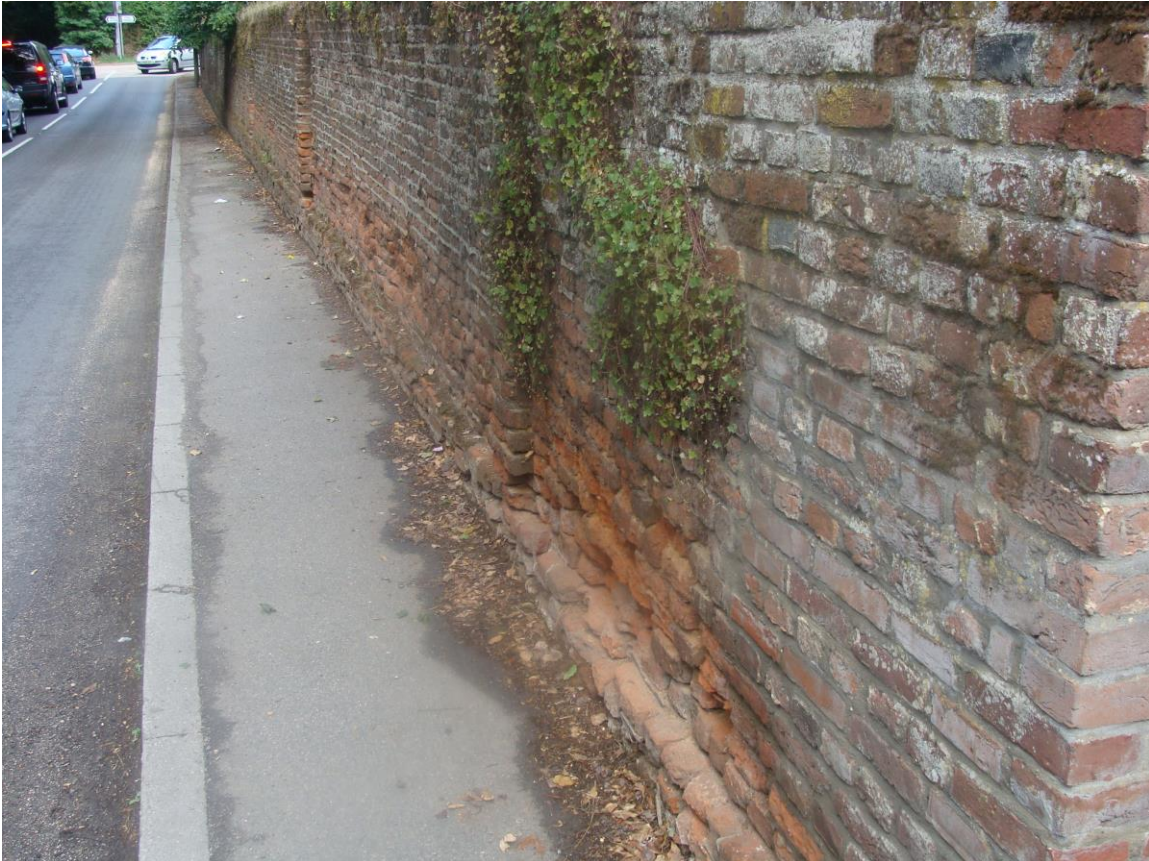
Picture 13- Grade II boundary wall, The Lordship, in need of repairs.
