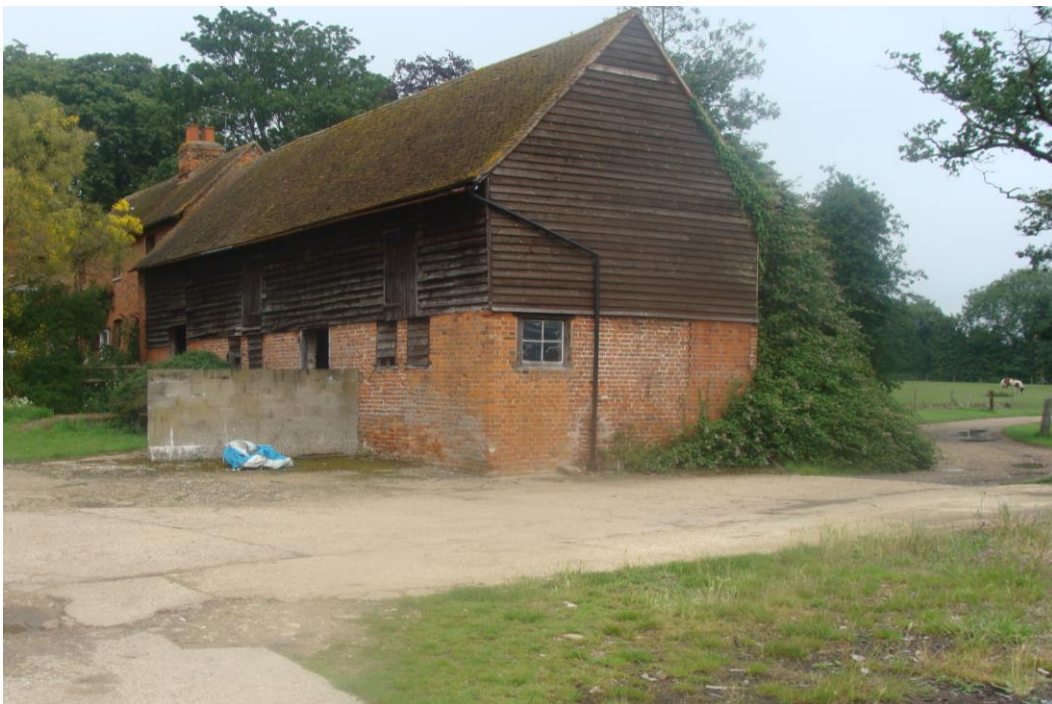
Picture 39- Agricultural barn at Moor Place in need of repair, damaged brickwork possibly caused by subsidence.
