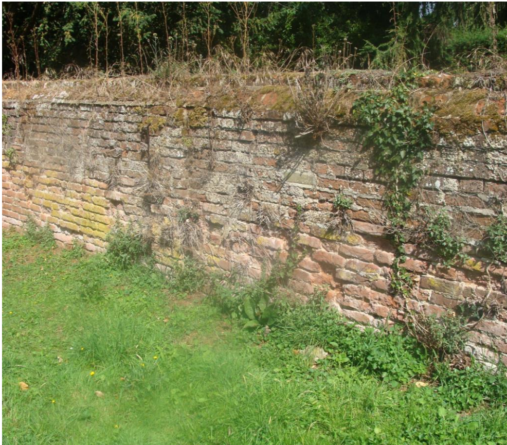
Picture 14 - Grade II wall enclosing churchyard, in need of repair and removal of vegetation.
