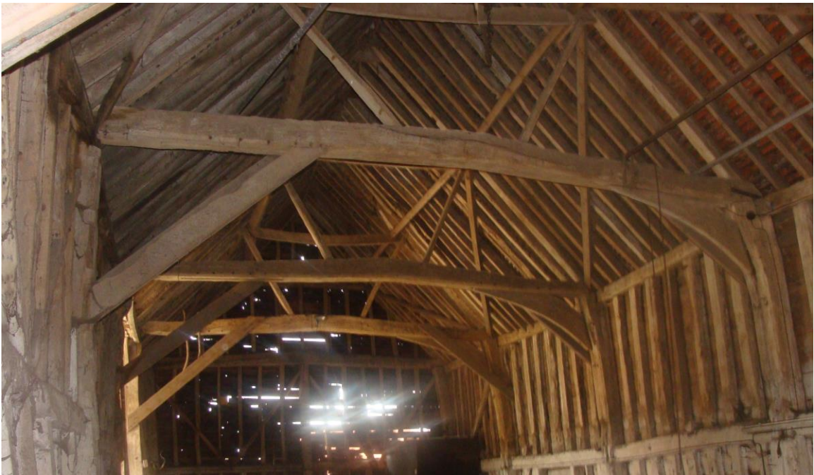
Picture 42- Same agricultural barn as previous, interior view showing construction post detailing, possibly dating from 17 th century in part.
