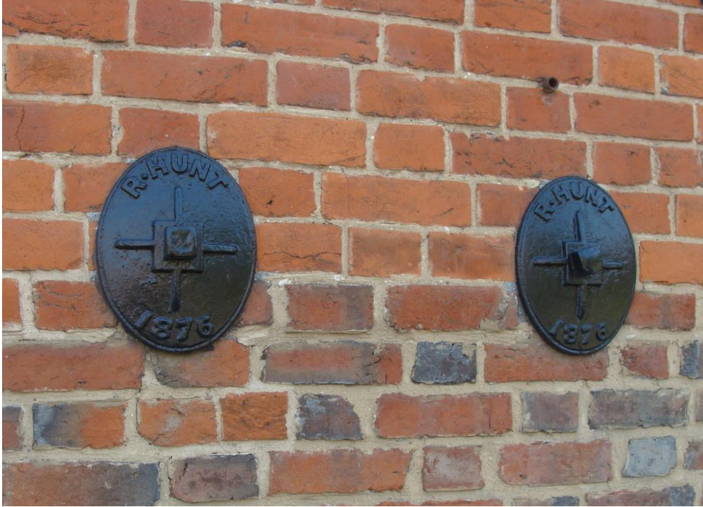
Picture 16- Tie rod plates to Culver Lodge, presume inserted at later date to rectify a 19 th century construction issue. Manufactured at the former Atlas Works, Earls Colne, Essex.
