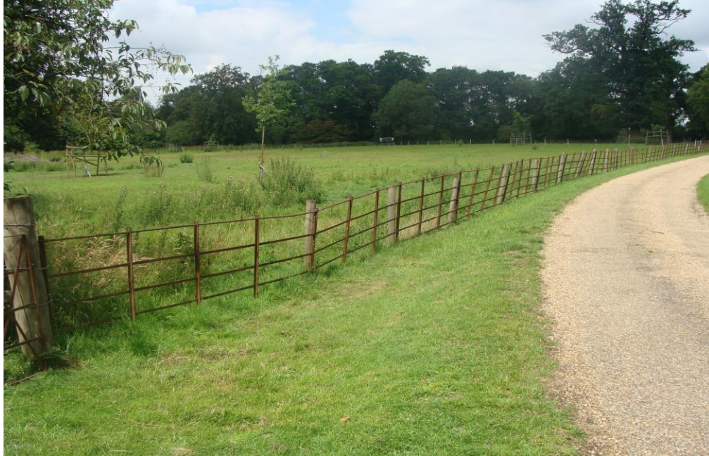
Picture 45- Typical late 19 th /early 20 th century agricultural fence at Moor Place, worthy of retention and in need of minor repairs.
