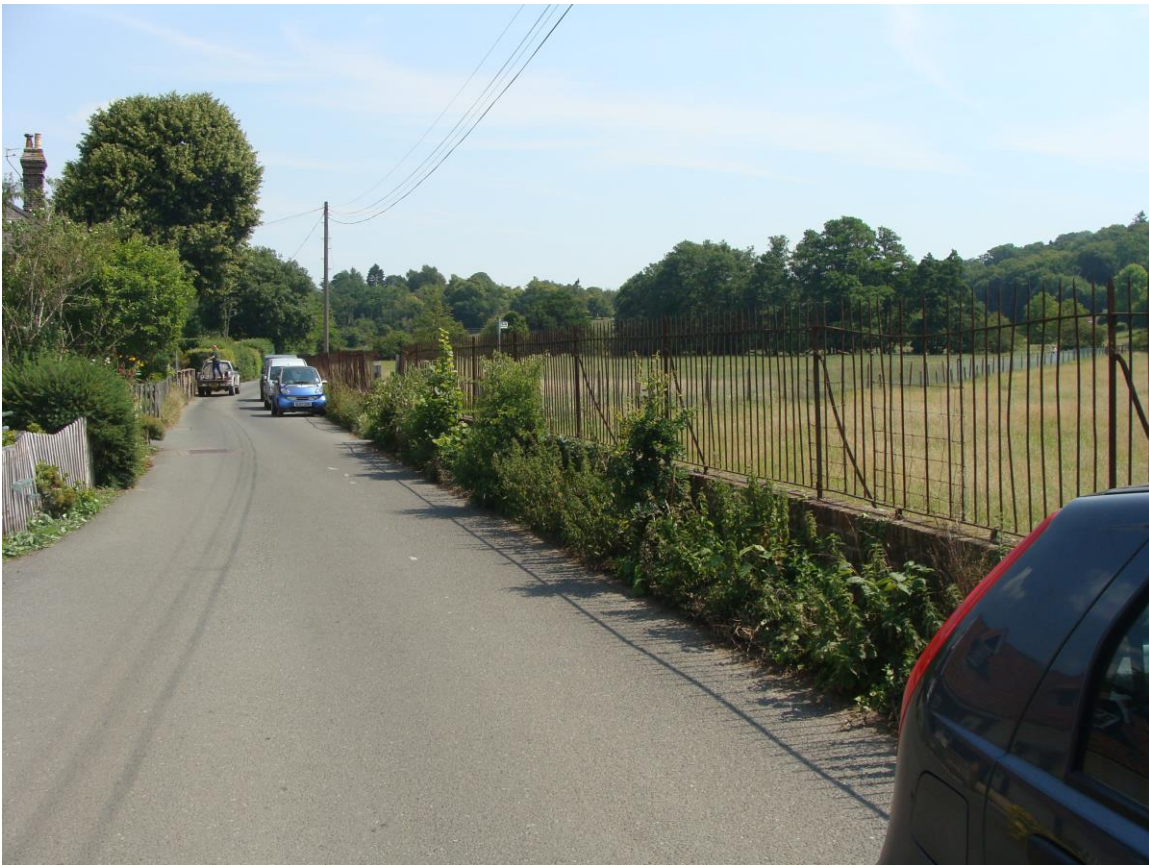
Picture 31- very long run of distinctive estate wall and railings, dating from late 19 th /early 20 th century. Some sections are in need of repair and/or replacement.
