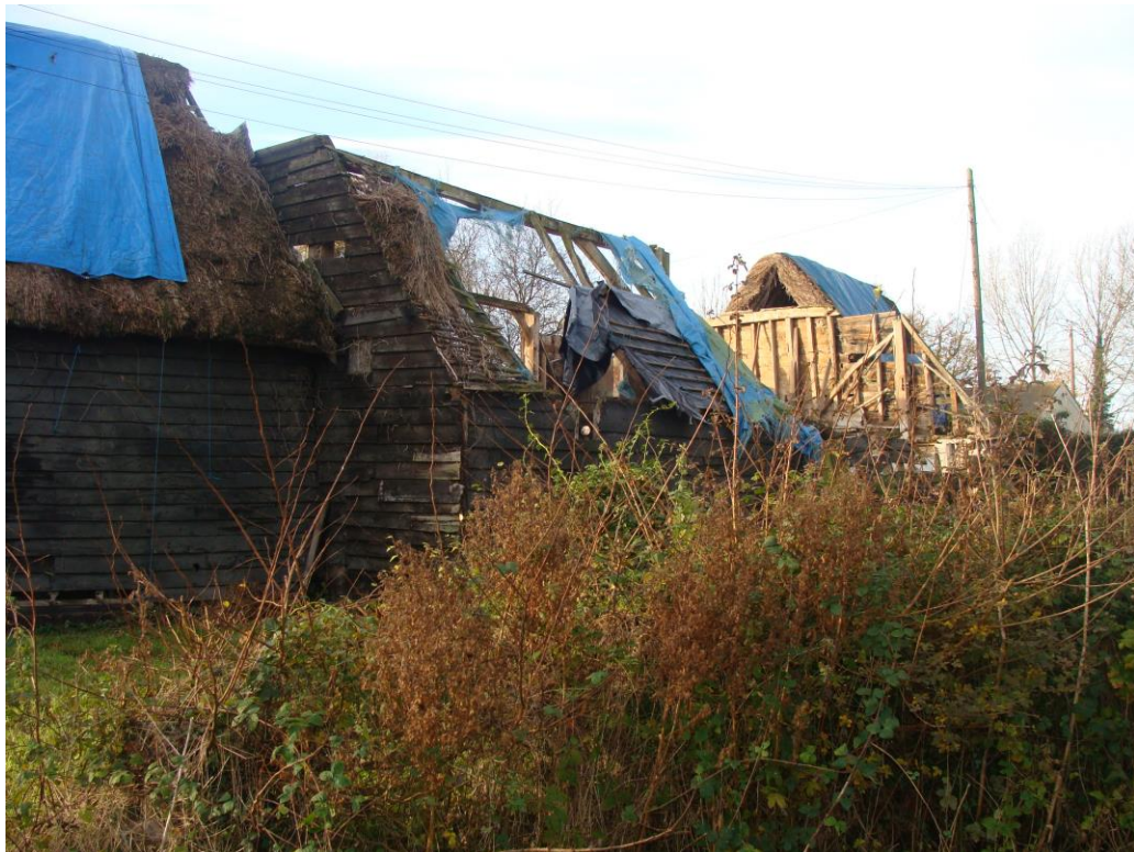
Picture 35 – Listed Buildings at Green Street in extremely poor state of repair. Discussions with owners of such properties are proposed to seek appropriate restoration.
