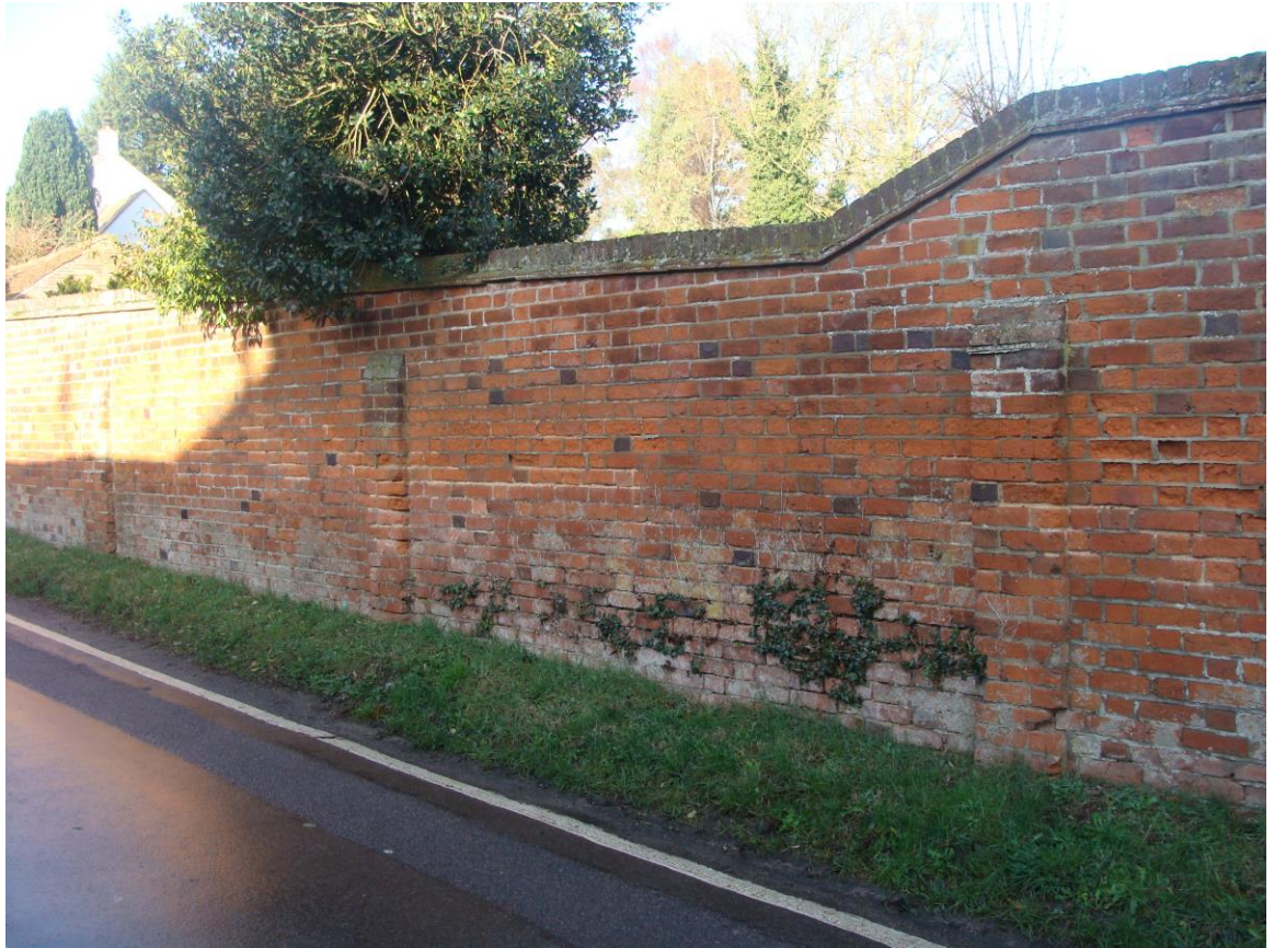
Picture 14 – 19 th century boundary wall to Ashford House at Chapel Lane, containing blue brick date detailing of 1869. Important wall in the street scene.
