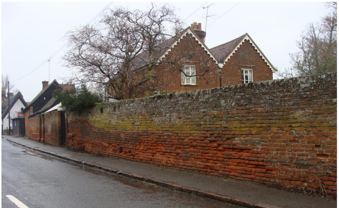
Picture 6 - Quality listed wall considered to be 'At Risk' and in need of repair.
