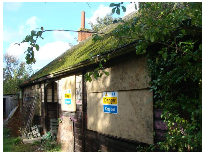
Picture 11. Building to south west of School House worthy of being returned to an appropriate productive use, subject to proper assessment and inspection.
