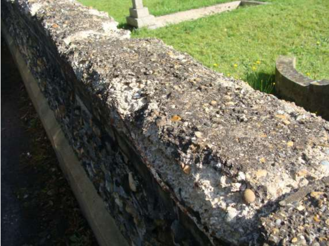
Picture 12 – Concrete capping slabs to church boundary wall. Picture retained as an historic record. These degraded capping slabs have now been replaced.
