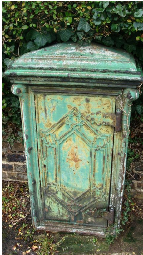
Picture 177. Unusual unidentified item corner of Ware Road/ Rowley's Road, possibly that of a utility company. Does the reader have any information?
