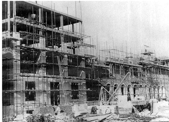
Picture 150. County Hall under construction in 1938. (Reproduced courtesy of Hertfordshire Archives and Records).
