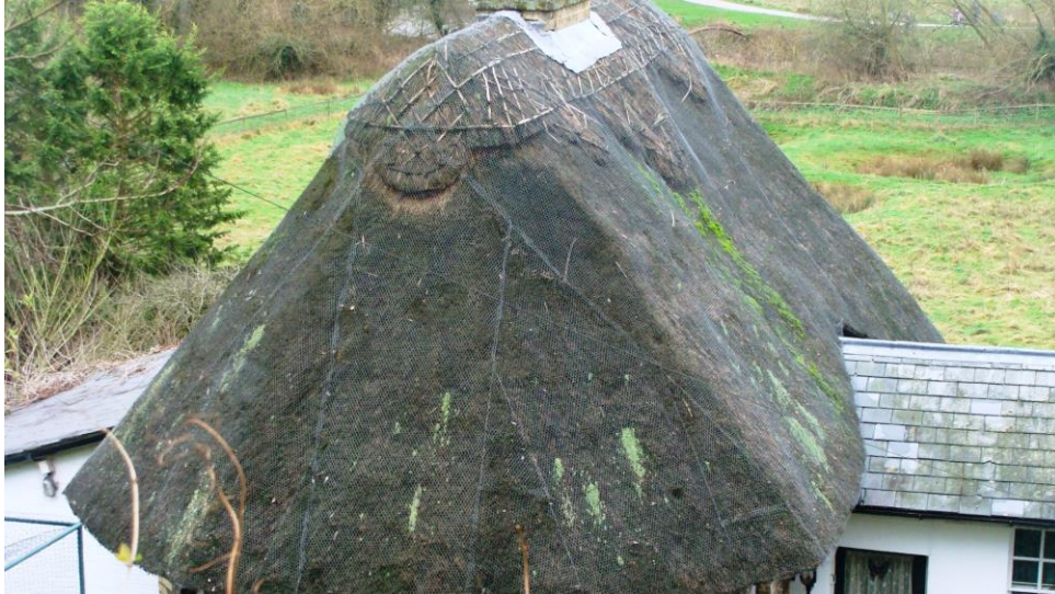
Picture 99. The Vineyard - thatched ridge appears in need of repair which may be eligible for EHDC grant assistance.
