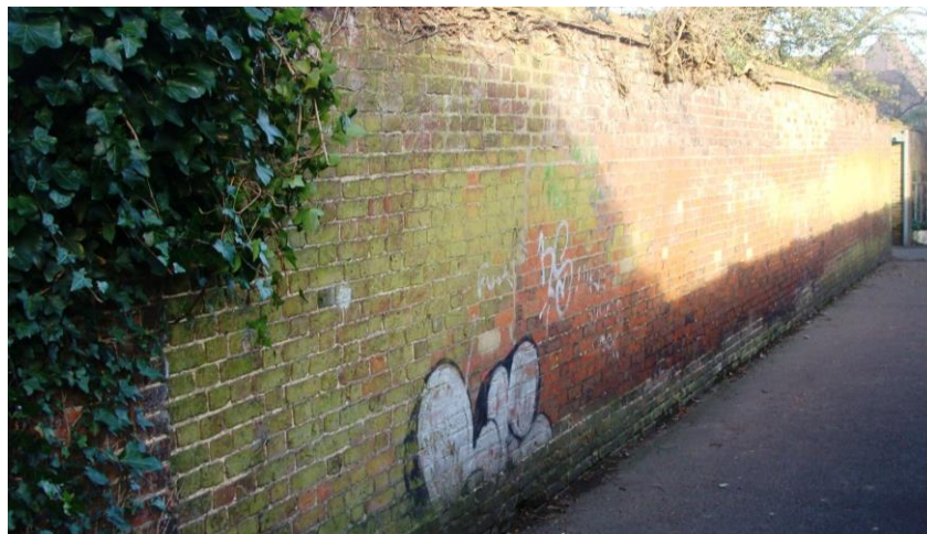
Picture 143. Wall forming boundary to Abel Smith playing field and adjacent to footpath need graffiti removing.
