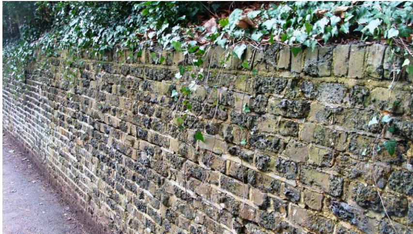
Picture 86. Interesting wall detailing on west side of Port Hill. Some bricks appear to be malformed with clinker residue attached.
