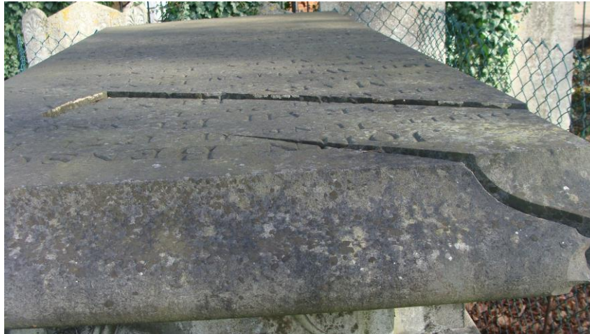
Picture 128. 18th century Benson tomb in need of repair. Now included on the Council's Heritage at Risk Register.
