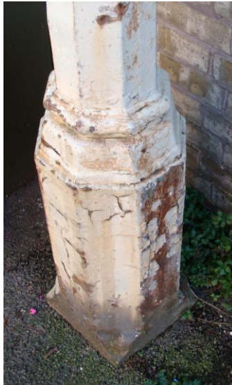
Picture 117. Detail of base of early street lamp on Chambers Street in need of refurbishment. Several of these have been noted.
