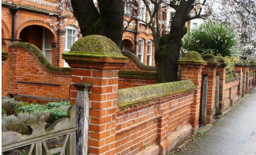
Picture 178. Good quality boundary and division walls to Nos. 111-115 Ware Road within the extended conservation area.
