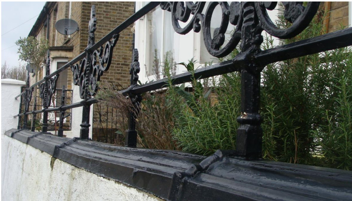
Picture 84. Very good quality early 20th century railings that are protected and which should be retained.
