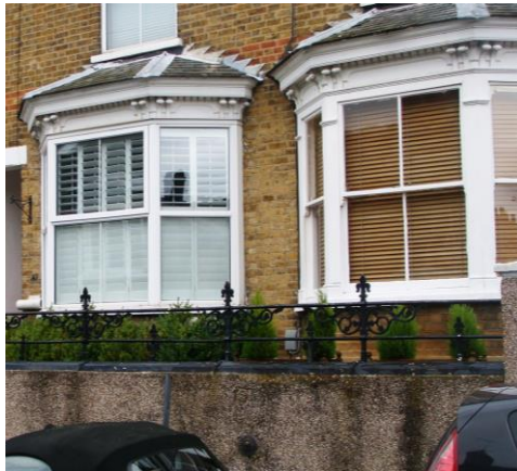
Picture 5. Window on the right is of traditional design; the replacement on the left is heavier and in comparison rather crude, in the fieldworker's opinion.
