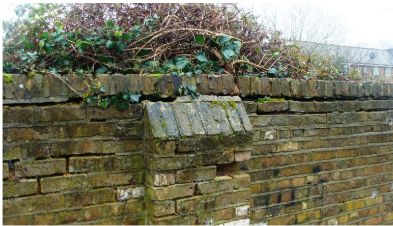
Picture 96. Wall at Pitteway Walk in need of repair.
