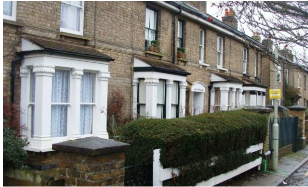
Picture 74. Distinctive window detailing to Nos. 37-43 Port Vale most worthy of retention.
