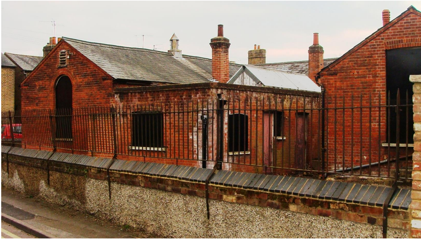
Picture 44. Part of a larger site at Dimsdale Street that is cause of concern and in need of further investigation before concluding its future.
