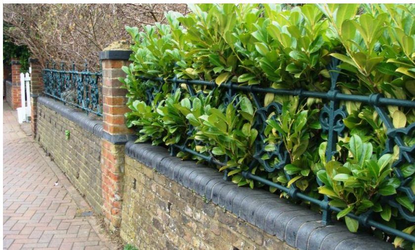
Picture 38. Good quality railings that extend along frontages of Nos. 60-90 Hertingfordbury Road.
