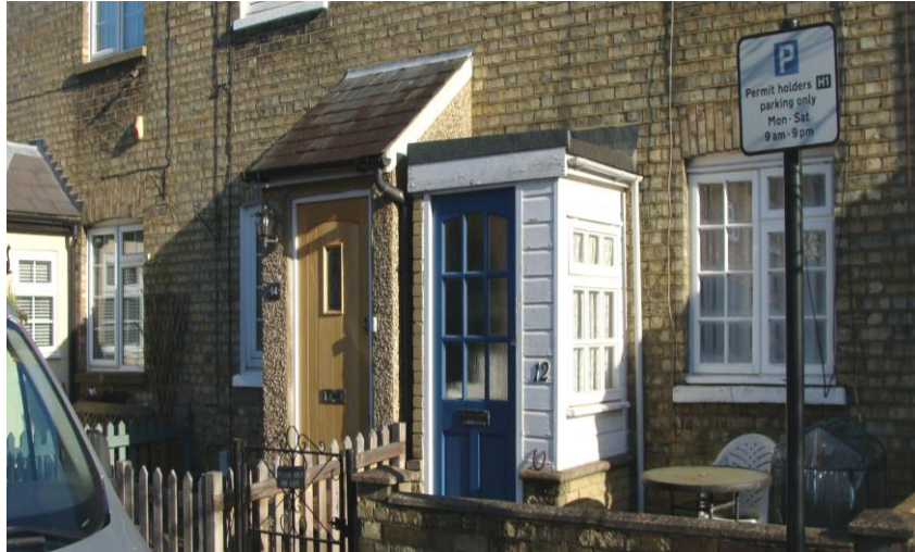
Picture 8. Inappropriate porch detailing.
