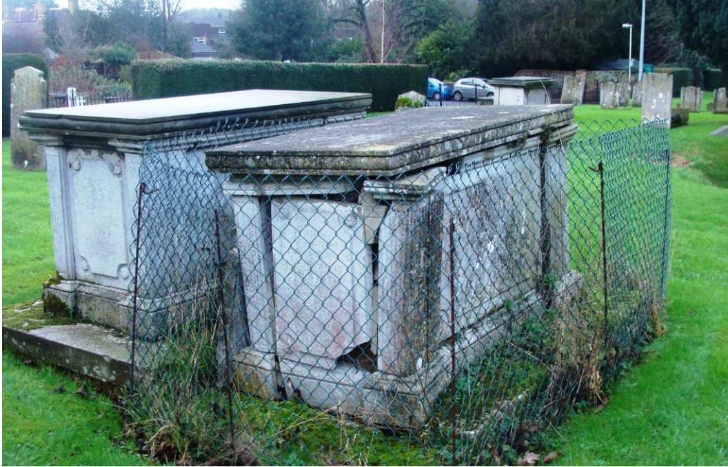
Picture 125. Damaged chest tomb at St. Leonard's churchyard in urgent need of repair which may be eligible for grant assistance from EHDC.
