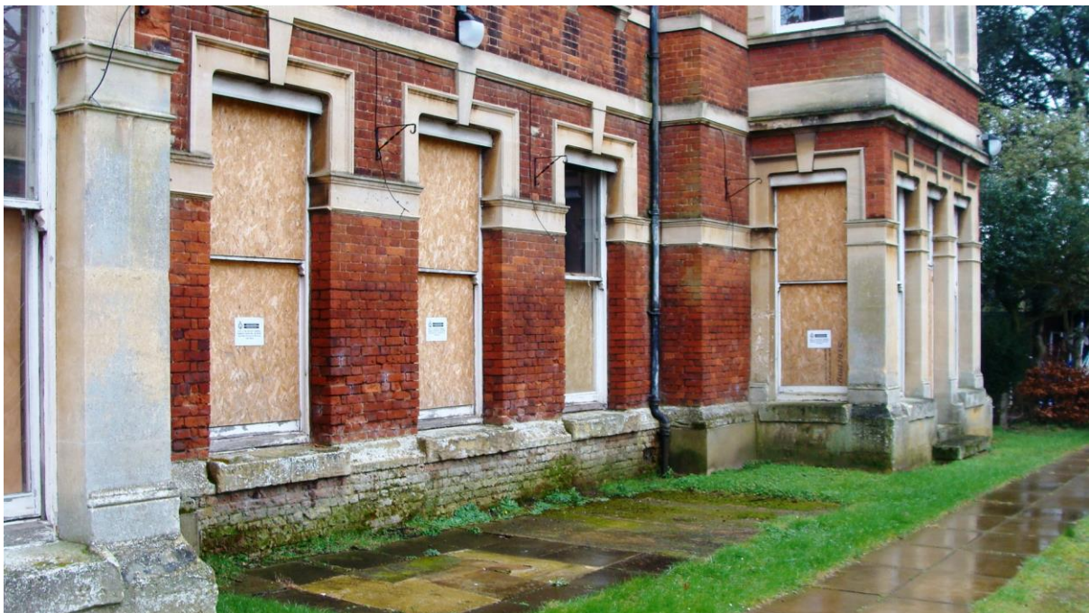
Picture 152. Leahoe House within the County Hall complex. A fine 19th century building in declining condition whose retention is important and whose future needs ascertaining.
