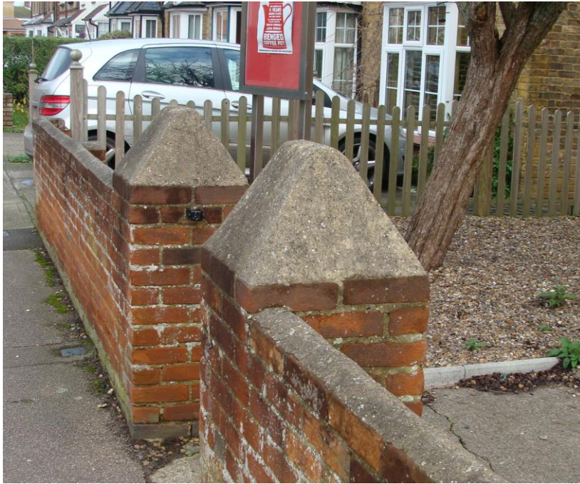
Picture 79. Brick wall to front of Bengoe Parish Hall which on balance is considered worthy of retention and additional protection subject to further consideration and notification.
