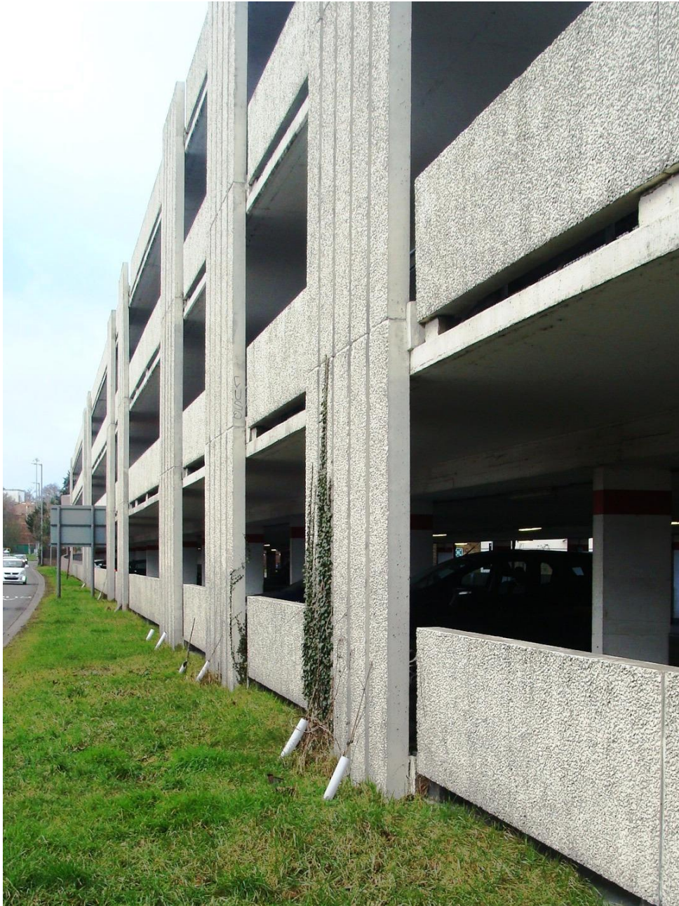
Picture 49. Attaining external professional advice to reduce the visual impact of Gascoyne Way car park is recommended.
