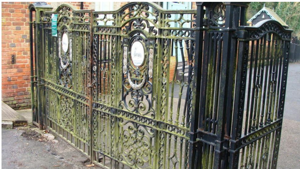
Picture 116. Decorative metal gates assumed to date from the earlier part of the 20th century are imposing and a strong feature in the street scene. Minor remedial works required.
