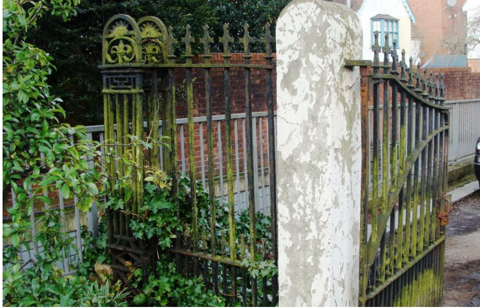
Picture 48. Listed gates etc. end of Church Street in need of refurbishment.
