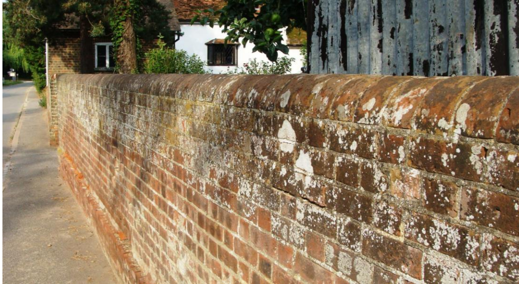
Picture 12. Wall to front of Little Meadow - a distinctive and attractive feature in the street scene.
