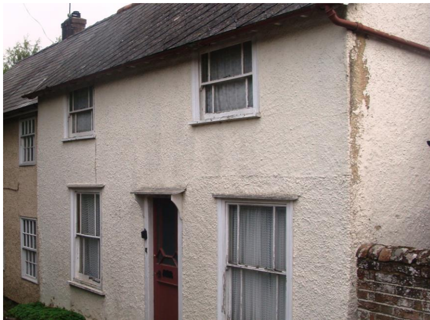
Picture 6. Cosy Cottage - the building is on the Council's Heritage at Risk Register and as such potential grant assistance may be available.
