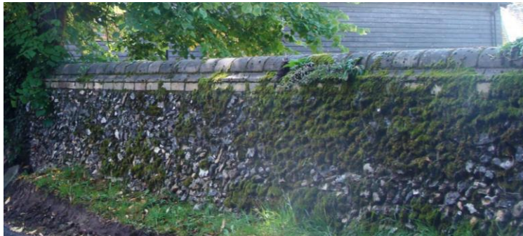
Picture 13. Wall north-west corner of Horseshoe Hill; prominent feature in the street scene.
