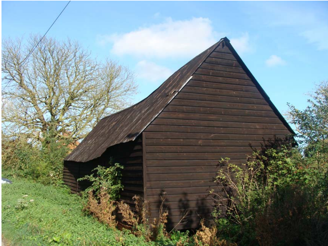
Picture 10 - Barn on east side of Ducketts Lane to south of Stuart Cottage. Its pleasing traditional form makes a positive contribution to the street scene and it should be retained.
