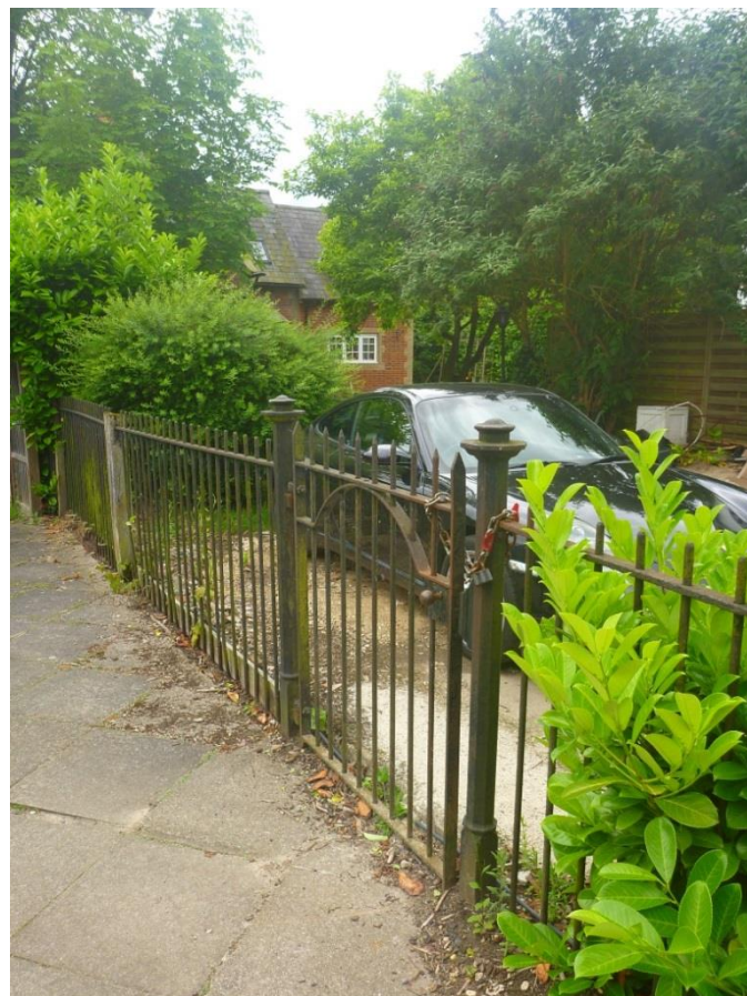
Fig. 54: Cast iron railings and gates on the West side of Furneux Pelham C of E Primary School. They are in need of maintenance and painting.
