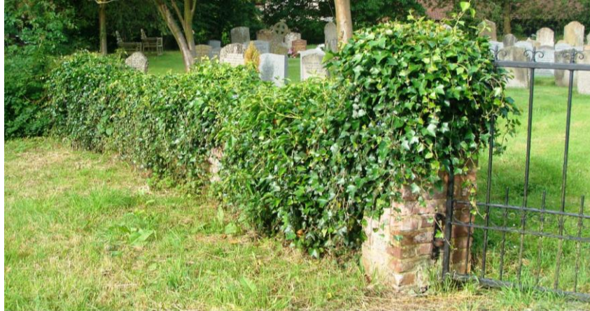
Pictures 22-23. The varied characteristics of the boundary wall to the church. Some repair work needed associated with selective removal of ivy.
