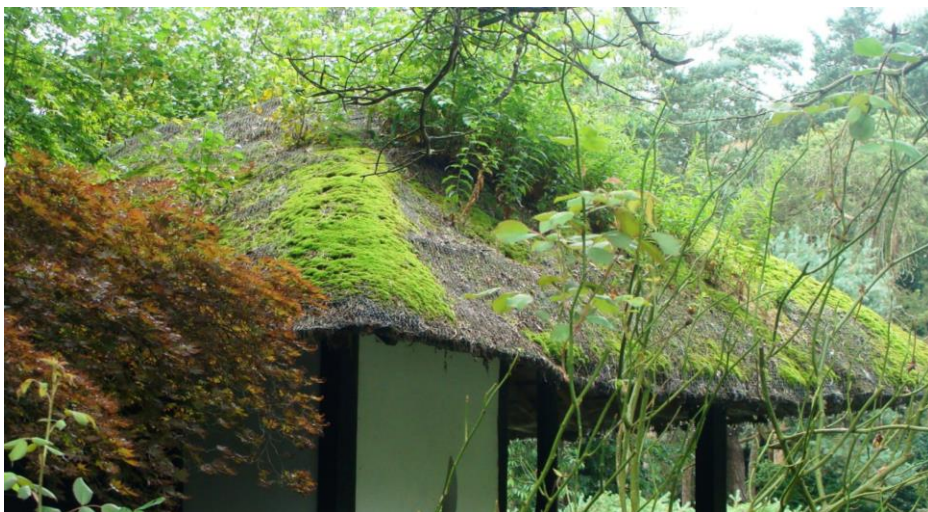
Picture 2. A listed structure in the Japanese Garden with deteriorating thatched roof; a candidate for the Council's Heritage at Risk Register subject to further investigation. This building was observed and photographed from adjoining Cheynes House.
