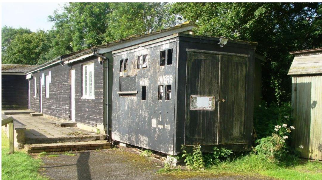
Picture 44. The cricket pavilion and associated facilities would benefit from improvements.
