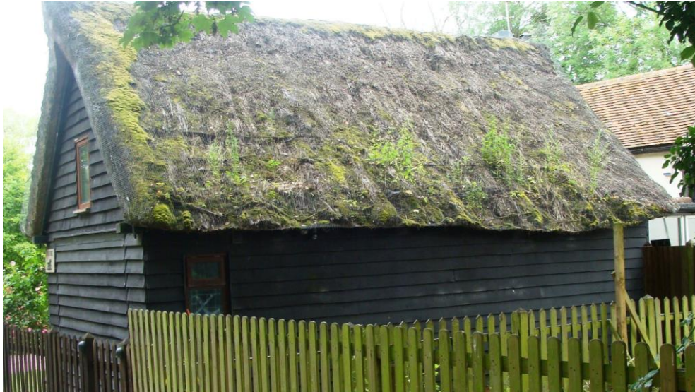
Picture 13. Ancillary building to the Old Forge whose thatched roof needs attention.
