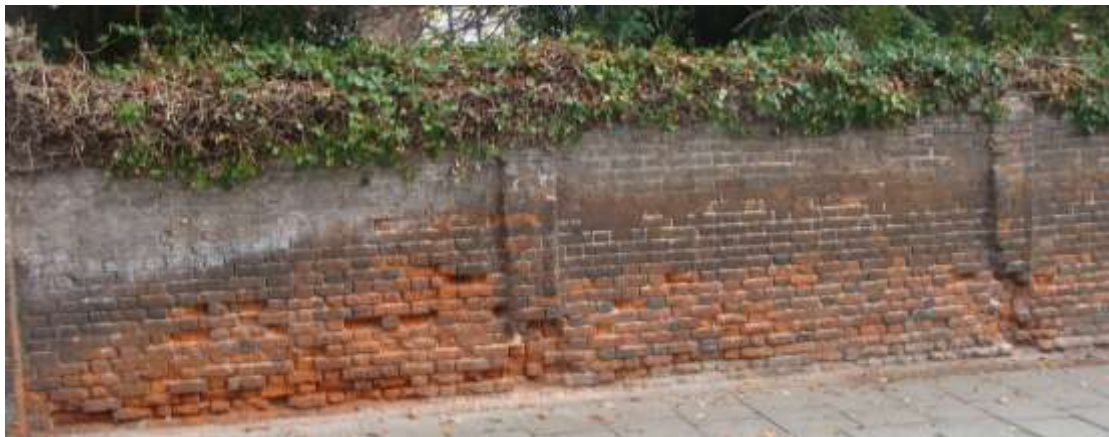
Picture 41. Wall to frontage of Old Grammar School in urgent need of repair and potentially eligible for grant assistance from EHDC. Wall now removed, photo retained in document as record.
