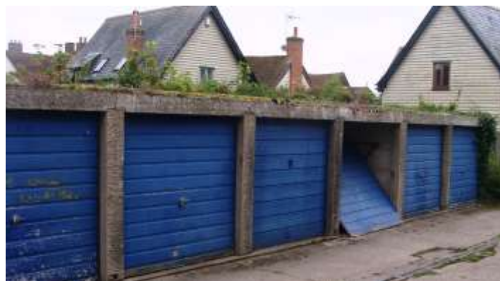
Picture 55. Poor quality lock up 'garaging' area that detracts. They are now removed from the Conservation Area. Can any improvements be made. What is its future?
