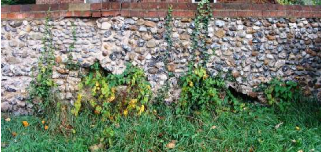
Picture 45. Boundary wall to New Cottage, The Causeway in need of repair and removal of vegetation.
