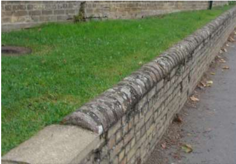
Picture 44. Curtilage listed low wall to Bridgefoot House. Modern concrete capping detail needs replacing.
