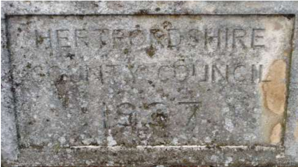
Picture 42. Plaque on bridge over River Rib needs re-inscribing to retain information for the future.
