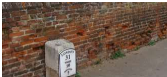
Picture 7. Repairs to spalled brickwork to St Peter's church may be eligible for grant assistance. Note the Milestone is also individually listed (the new metal plaque was attached in 2006).
