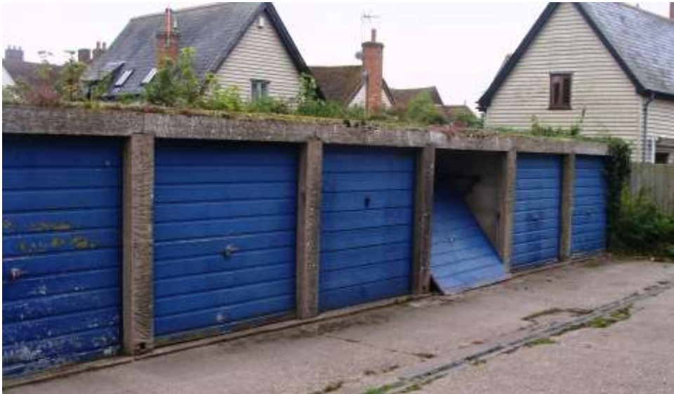
Picture 68. Garage block now removed from the Conservation Area. Notwithstanding this improvements are needed.
