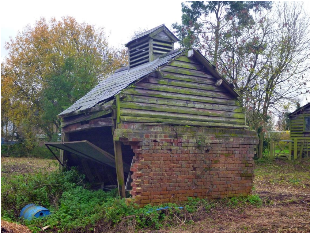
Fig. 59: Dilapidated building behind Hall Farmhouse.
