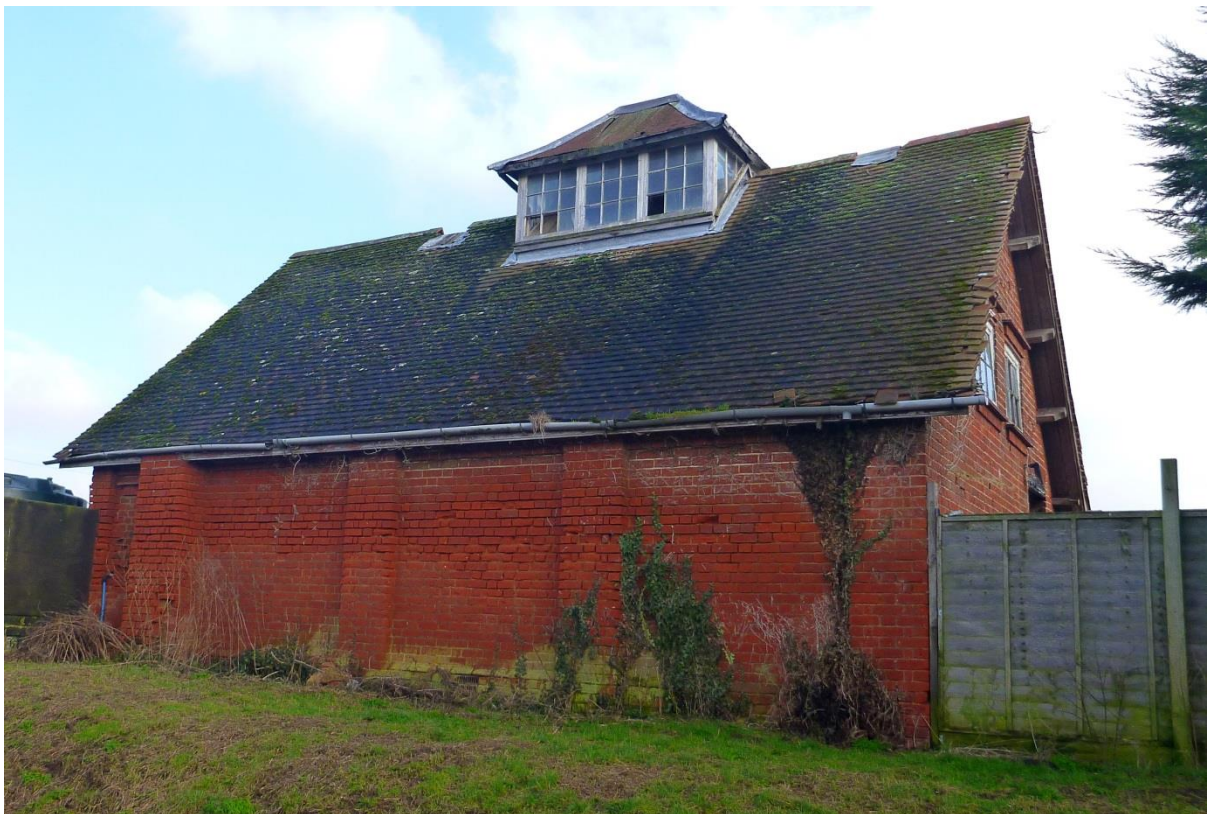
Fig. 23: Interesting outbuilding at The Kennels in a poor state of repair
