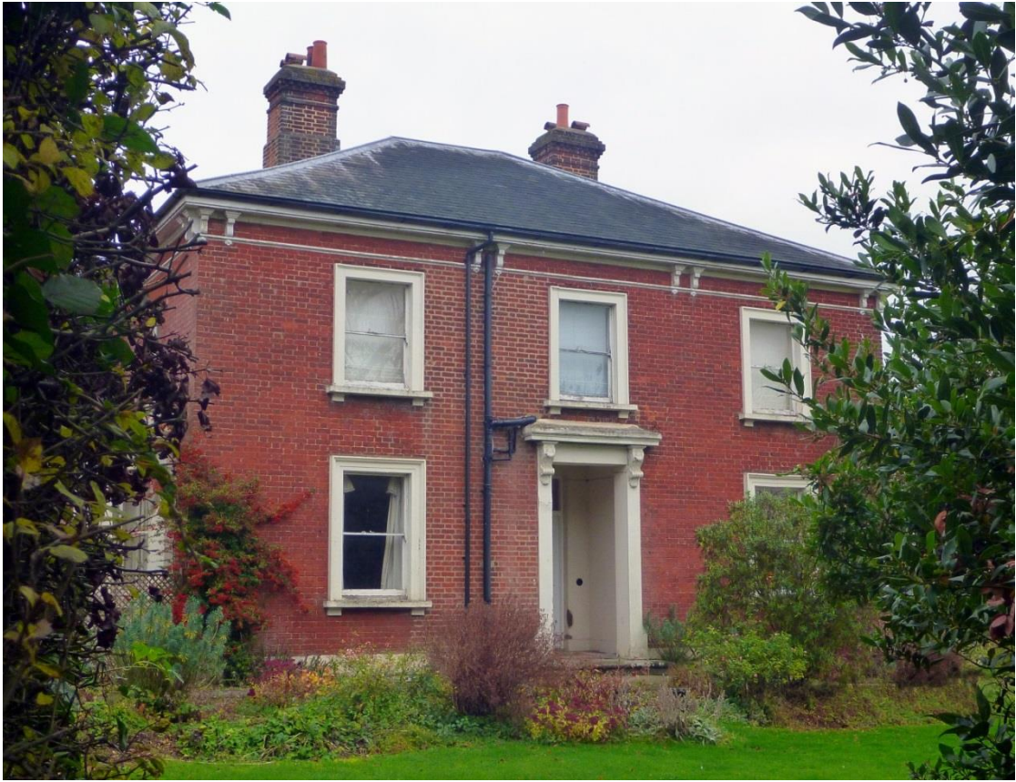
Fig. 36: Hall Farmhouse. An attractive mid-C19th building but it would be improved by the removal of the exterior pipework on the principal elevation.
