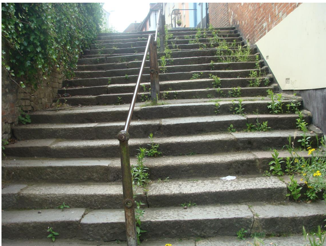
Picture 97. Flight of steps and railing, probably from 19 th century in need of renovation; minimal work relating to removal of vegetation (as seen in this picture) has been carried out.
