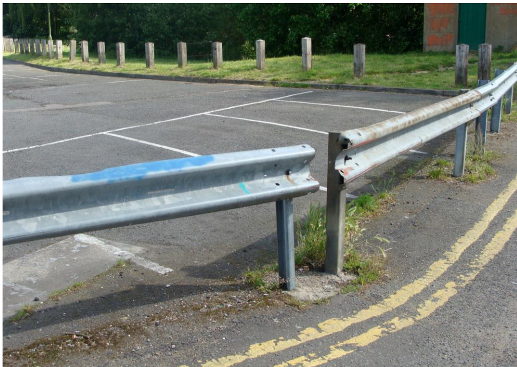
Picture 55. Disruptive former Metal barriers that were visually disruptive.
