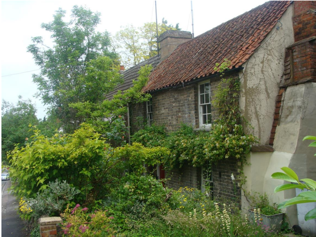
Picture 83. Nos. 10-12 Bell's Hill. Pair of non listed cottages worthy of retention. Some repair works to roof have been carried out.
