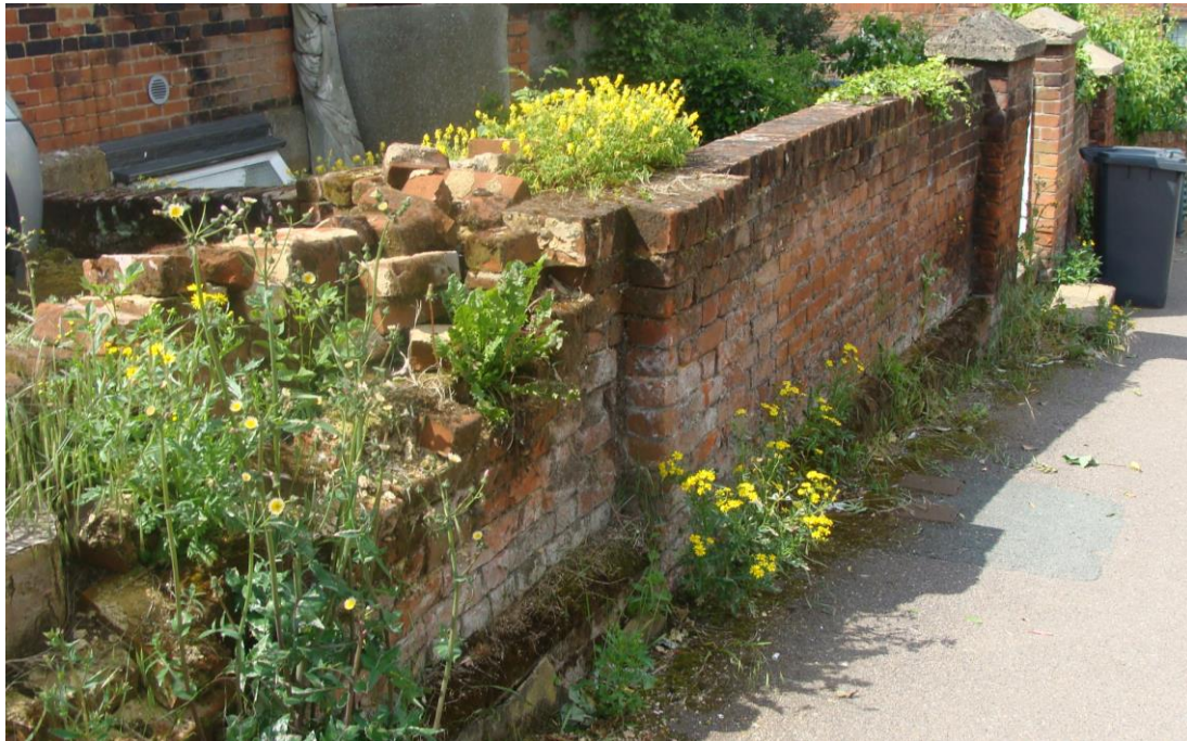
Picture 42. Wall at Grange Road in urgent need of repair.
