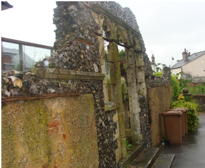
Picture 77. Listed Building entrance arch to no. 5 Half Acres, a Listed Building at Risk and in urgent need of repair and consolidation.
