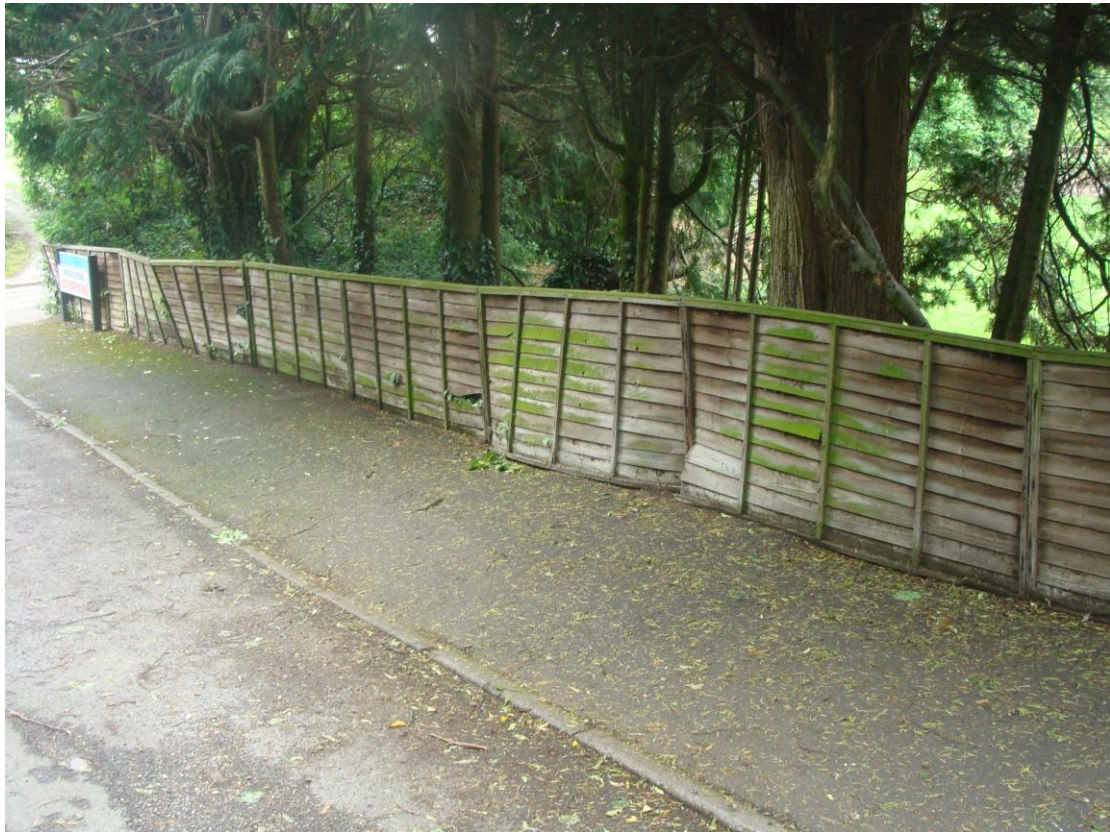
Picture 17. Deteriorating fence to front of Snowlands. This may need replacing in the future; an ideal solution would be with railings or hedge.
