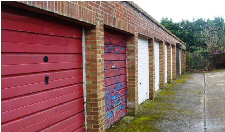
Picture 31. Garaging area north end of Stringers Lane would benefit from general improvements including co-ordinated paint of garage doors.
