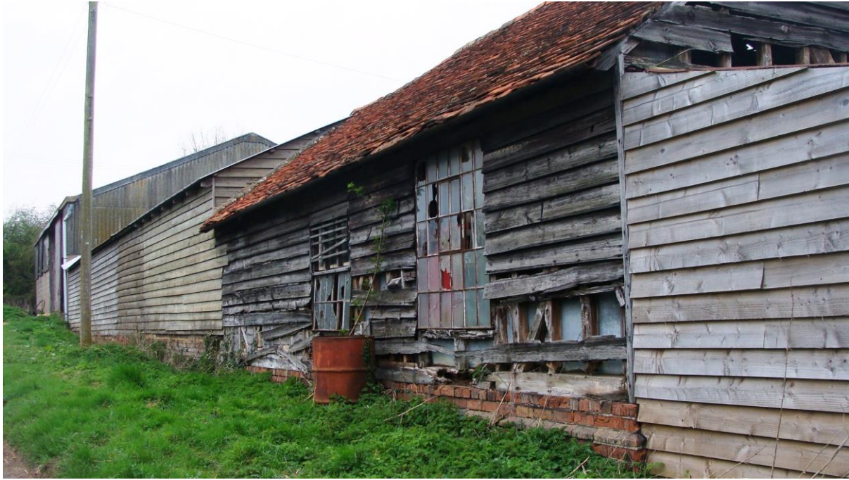
Picture 43. Buildings interpreted as curtilage listed at Coates Manor Farm on the Council's Heritage at Risk Register in urgent need of repair on this important approach to the village.
