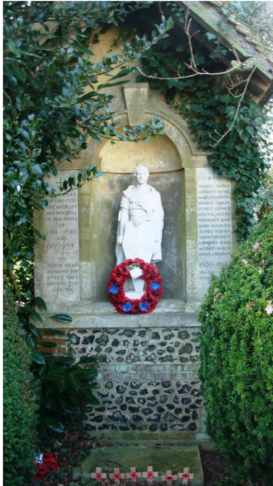
Picture3. War Memorial- a most unusual design. Removal of selected vegetation would be advantageous. The fieldworker was advised the central figure of St George is a replacement following theft of the original.
