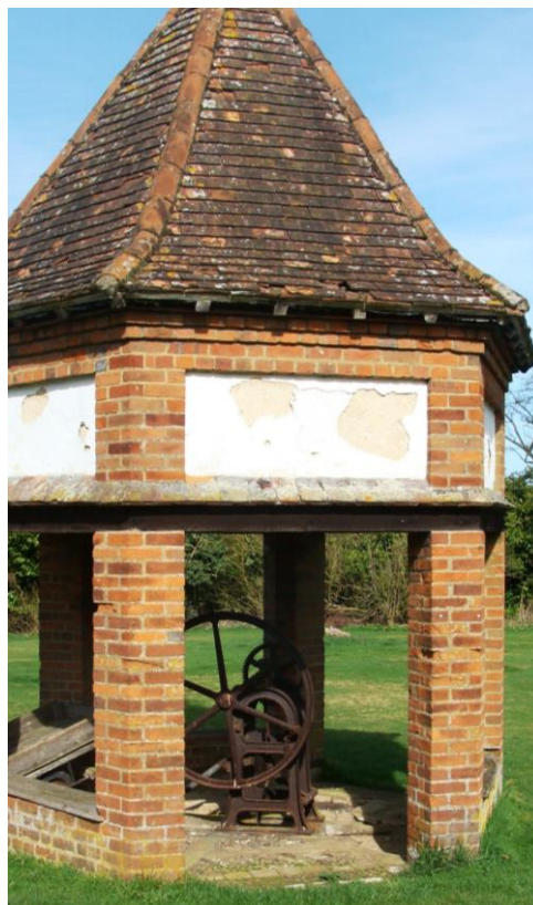
Picture 4. Village pump and well house. Simple repair works at modest cost would result in significant improvements. Without prejudice financial assistance may be available.
