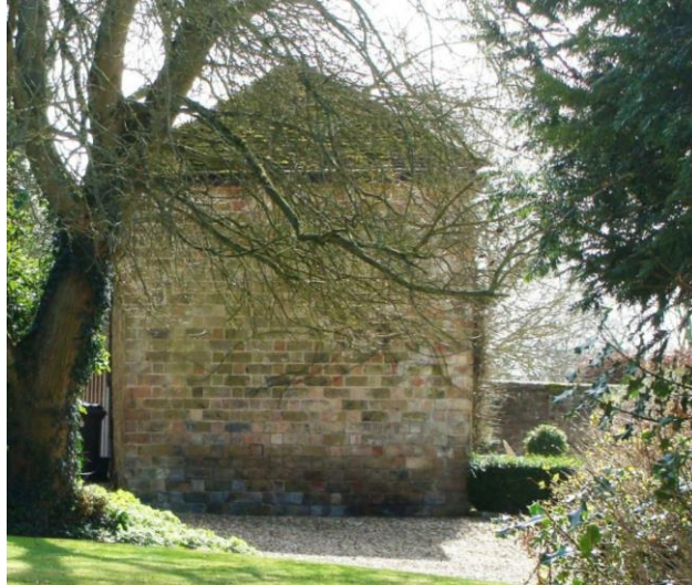
Picture 6. Ancillary building in the curtilage of The Old Vicarage, viewed from road. Unusual brick construction - Rat Trap bonding.
