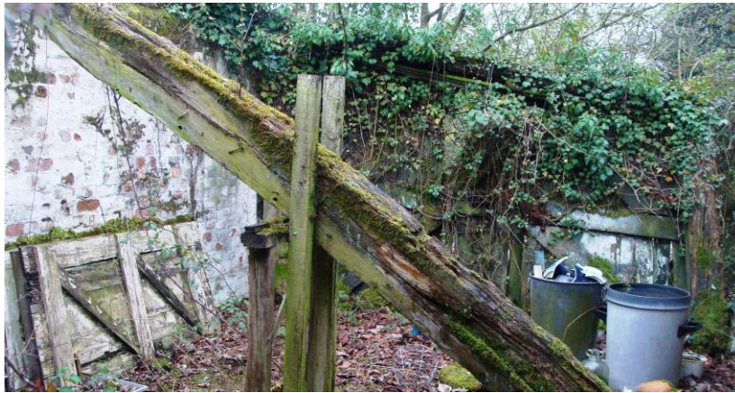
Picture 42. Ancillary curtilage listed building within curtilage of Spring Grange that is in very poor condition. It has been on the Council's Heritage at Risk register for a number of years and this structure together with the main building (see above) continues to deteriorate.
